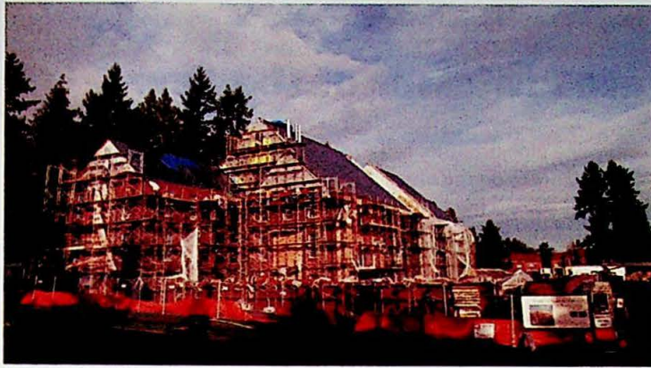
PROGRESS Part of the transformation at the south end of campus includes the demolition of South Hall and the construction, now underway, of the new Center for Health Sciences. This photo was taken in December. The building is on track for completion in the spring.
